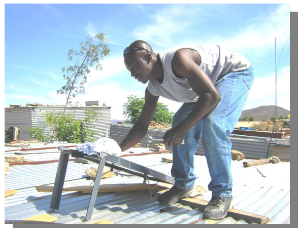
The cell phone charging system is powered by one small solar panel, which is easily removed at night and stored safely.
