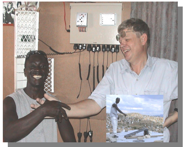
Venasius Amukwa's solar cell phone charging shop in Havana, Windhoek, has attracted a much attention from local and international renewable energy suppliers and organisations.
