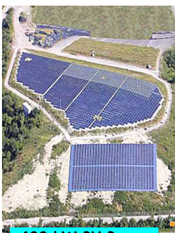
428 kW PV Power Plant, Germany
