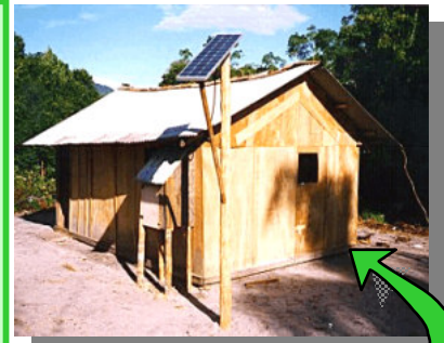
80 W (0.08 kW) Solar Home System
