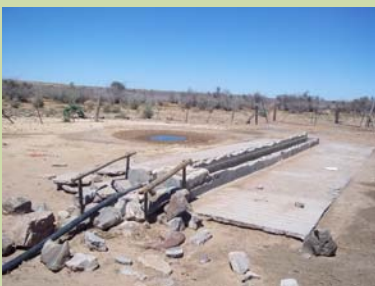
Damaged watering trough needing repairs to prevent water losses and pollution.
