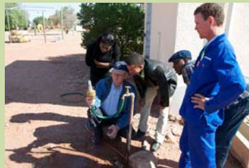
Support team discussing how to minimize leakage in water supply system together with representatives from Oskop Local Authority.
