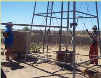
Assessment of water infrastructure on Odendaal farm in Hardap region, note the kraal just behind the borehole.
