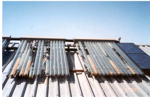
Figure 10: Broken vacuum tubes of TAS solar panel after a hail storm [Stöck, 2004]
