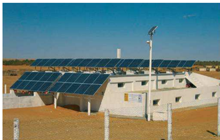
Figure 2: 10.5 kWp solar electricity-operated reverse osmosis of brackish water in Tunisia with a fresh water output of 15 m 3 /day [WISIONS, 2008]
