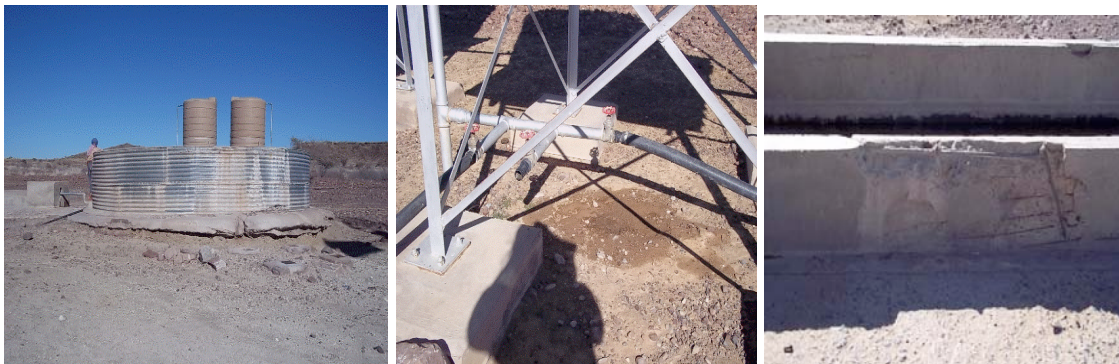
Figure 4 Natural and Infrastructural challenges (from left to right): soil erosion around dam, leakages, fragile infrastructure of water troughs
