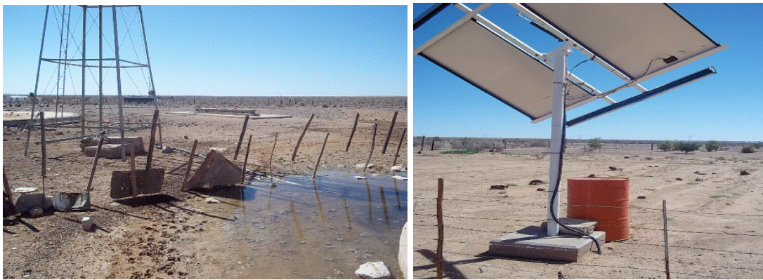
Figure 5 The unrehabilitated water point situated in the kraal area (left) and the solar-pumped borehole (right). The panel is within the fenced-in plantation site.
