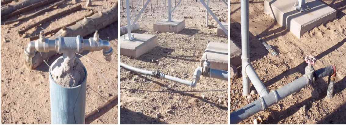
Figure 3 Maintenance is an issue in managing the water point, as depicted in the pictures, where a neglected standpipe with misplaced handles and exposed water pipes are visible
